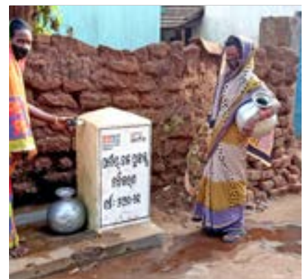
Su-Swasthya safe drinking water pipeline, Sukinda
